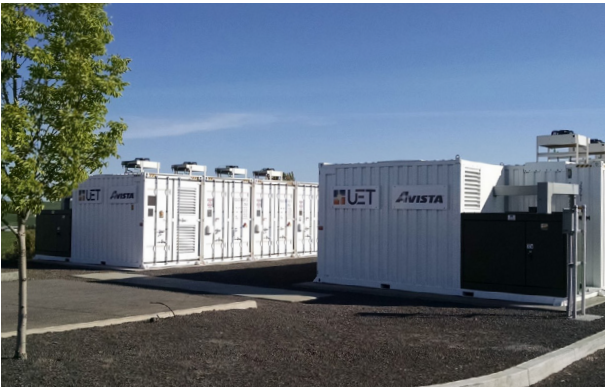
Example battery storage system
